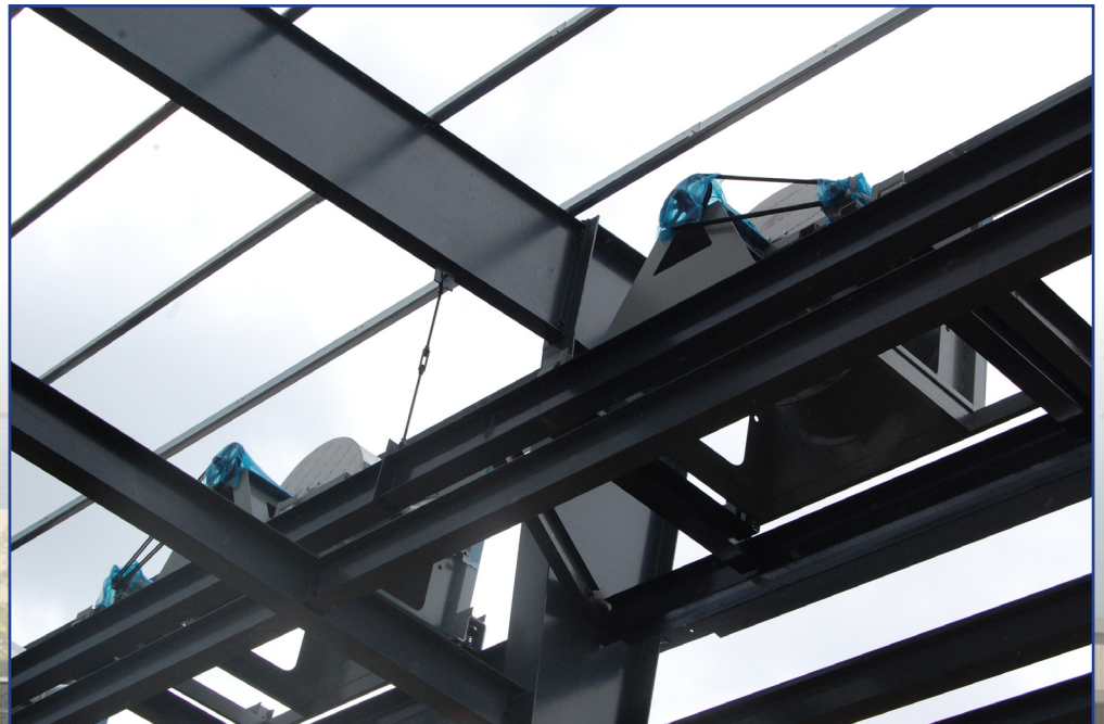
Right: There are 54 intake fans being installed for the state-of-the-art ventilation system.
